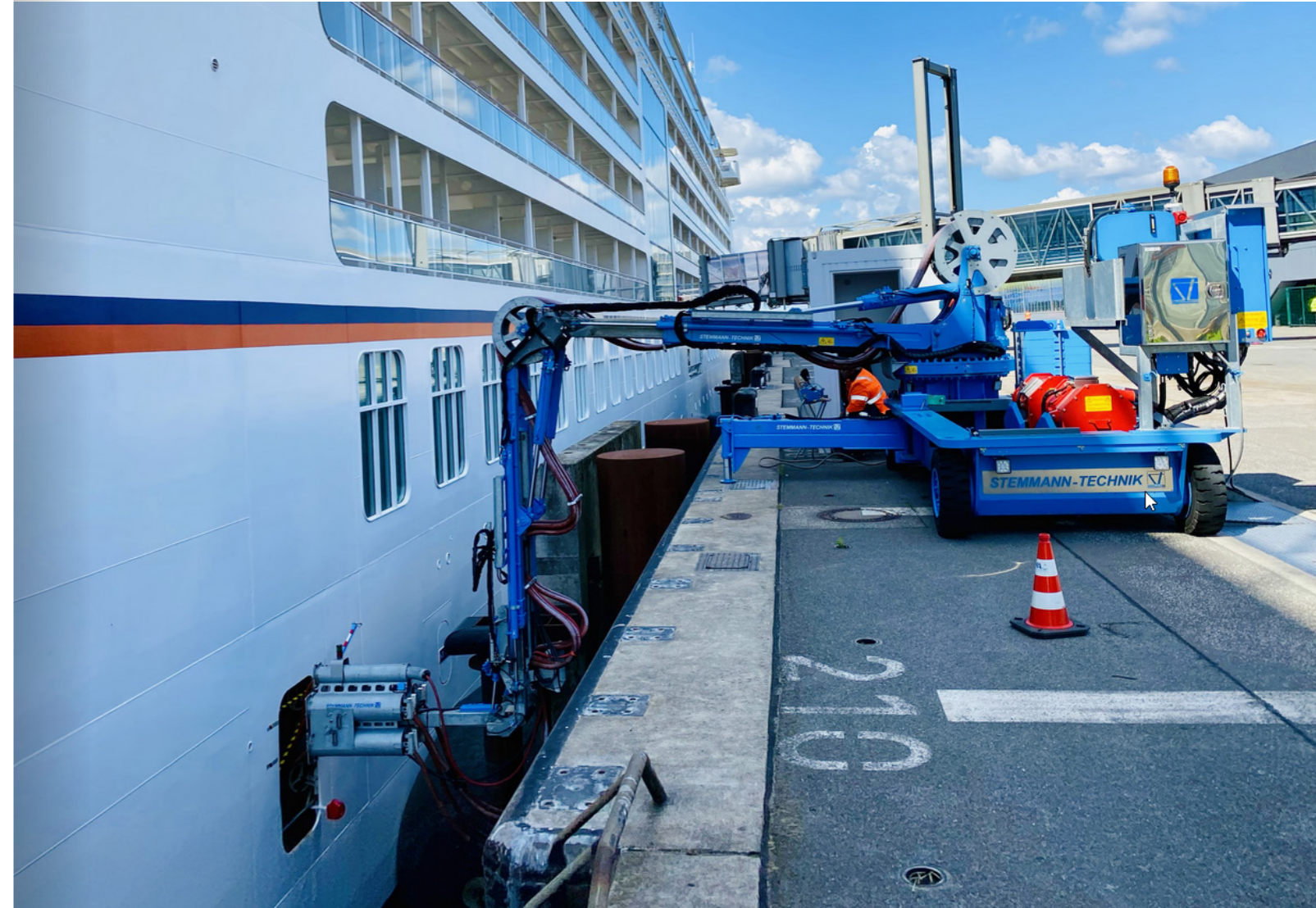
Figure 6.11 Onshore power supply for a cruise ship (source Stemmann-Technik)
